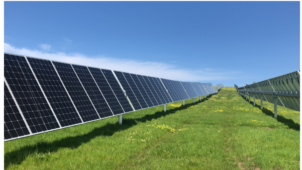
Figure 1. A close view of the solar panels on the farm
