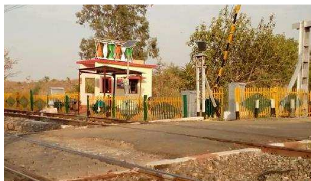
A 1.75 Kw installation on Railway Crossing
