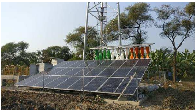
11Kw Installation for Telecom Tower
