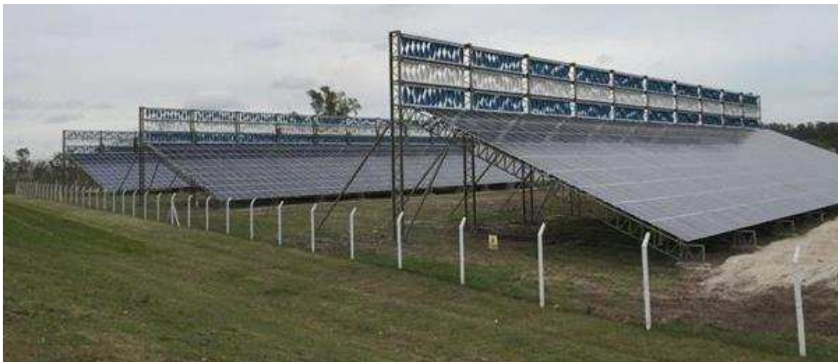
MW Scale Installations
