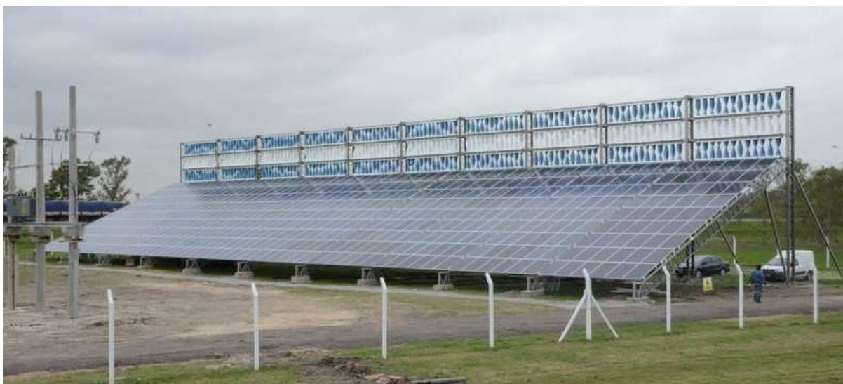
40Kw Power Mil installation for Mini Grid application.
