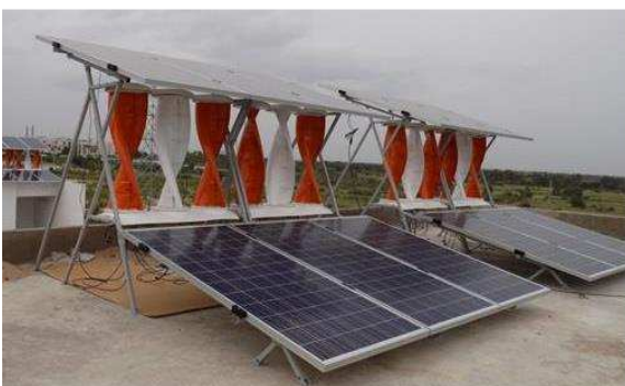
A 10 KW Hybrid Installation @ Industrial area Shammerpet, Hyderabad
