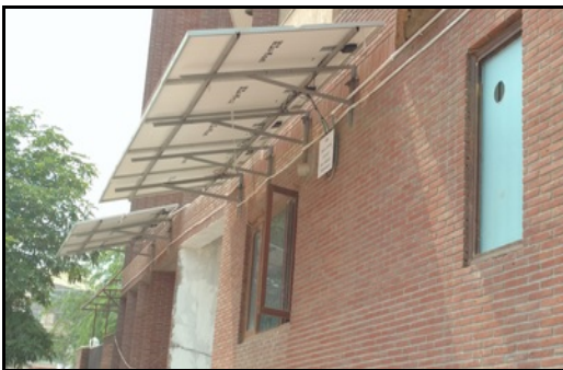
Implemented roof top Solar panel projects by Spectron Solar Organization
